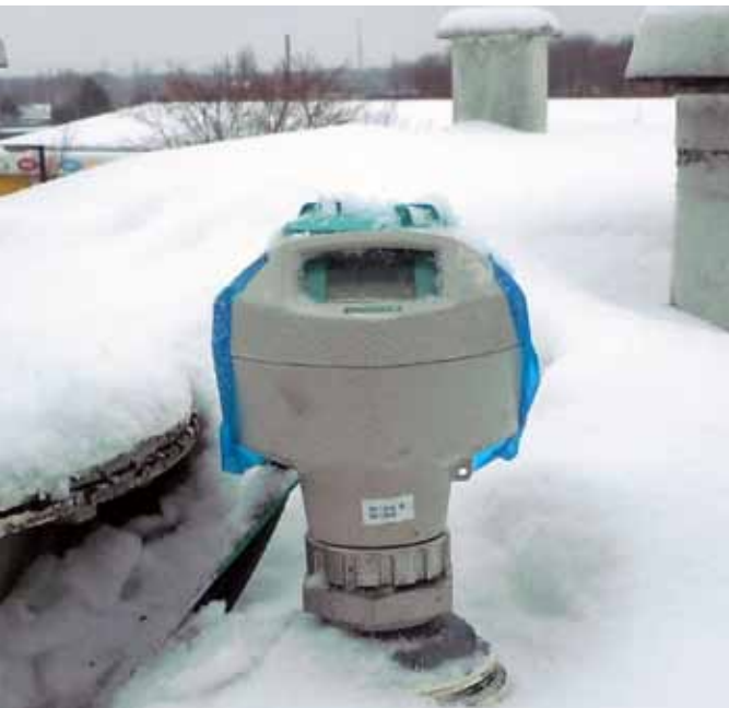
Installing the SITRANS LR250 was easy and the company now has reliable, high-performance continuous level measurements on their storage vessels.
