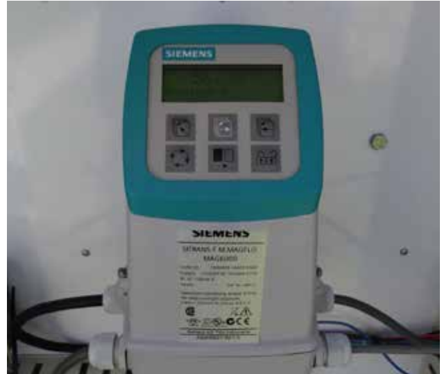
SITRANS F M MAG 6000 transmitter remotely connected to the 66-inch SITRANS F M MAG 5100 W flow meter sensor.
